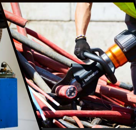
Cable Recycling & Production
